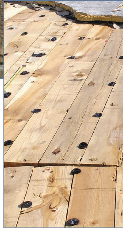
Photo 7: Edge flashing failure – SPF roof system depended upon attachment to rotten edge nailer.
