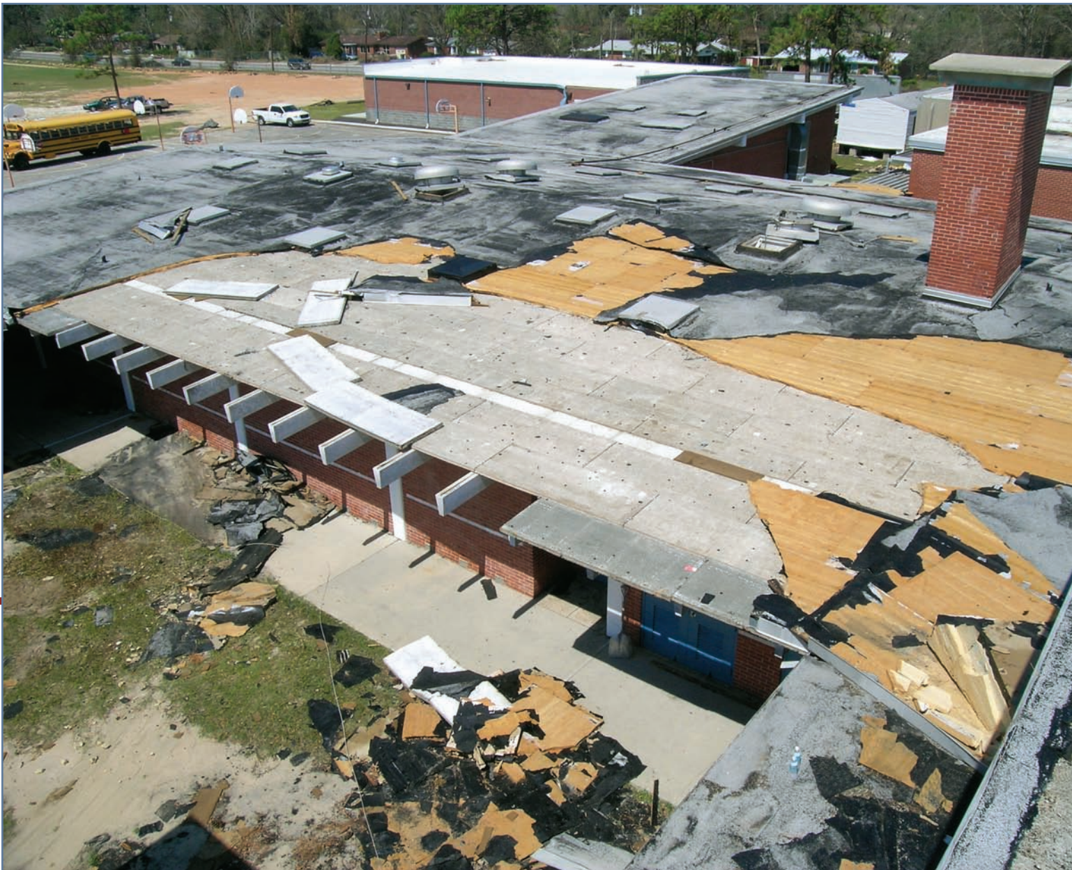
Photo 3: Overhangs increase uplift pressure. Special design is required.
