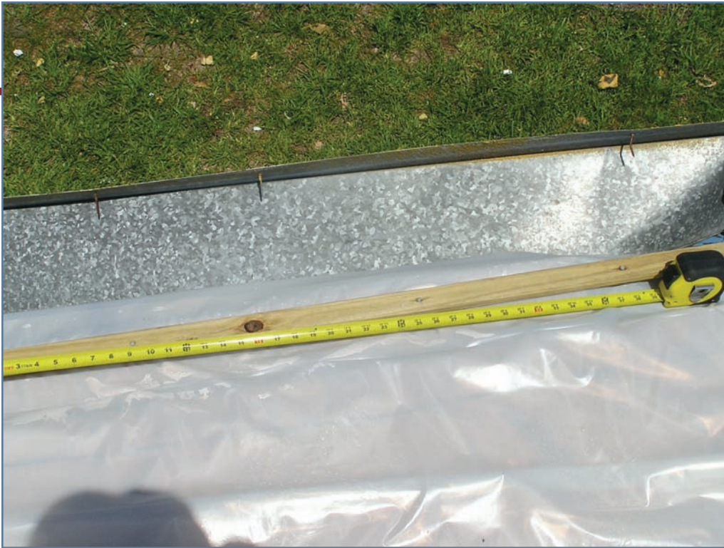
Photo 9: Edge flashing attachment – metal edge improperly fastened at up to 22" O.C.
