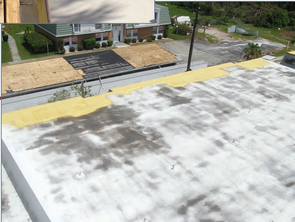
Photo 8: SPF edge repair – Adjacent BUR blew off, while the SPF roof only suffered perimeter damage due to inadequate nailing of metal edge flashing.
