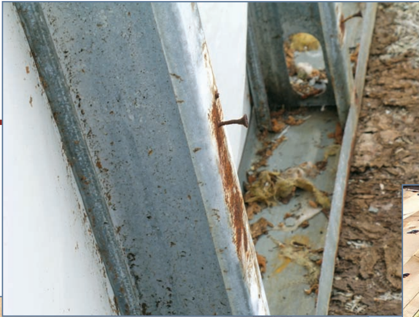
Photo 5: Corrosion is common in hurricane prone areas – especially near the ocean.
